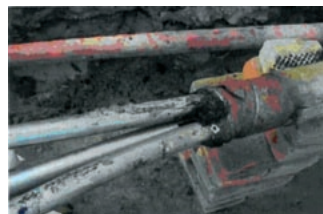
Fig. 2: Corrosion on the outer sheath and the building of holes in the lead sheath
