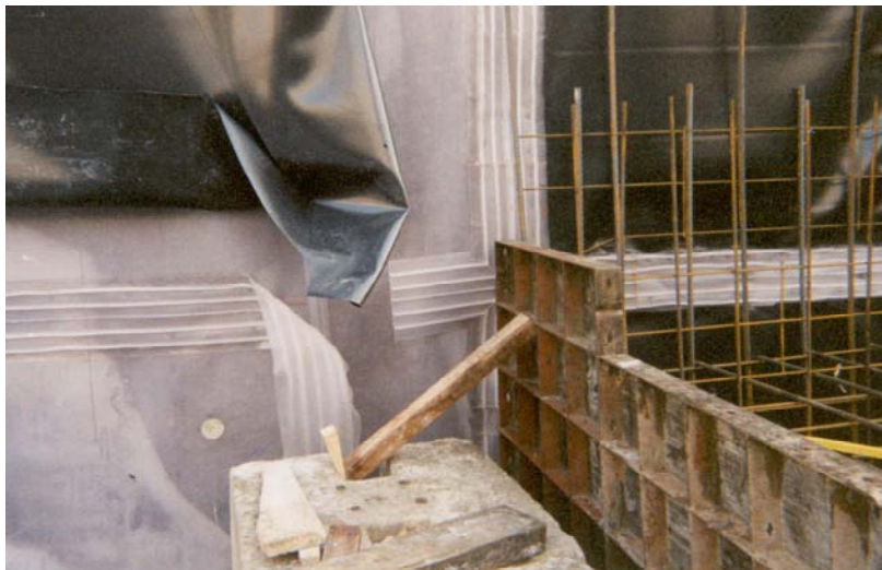
Dangers of mechanical impact to Waterproofing system
