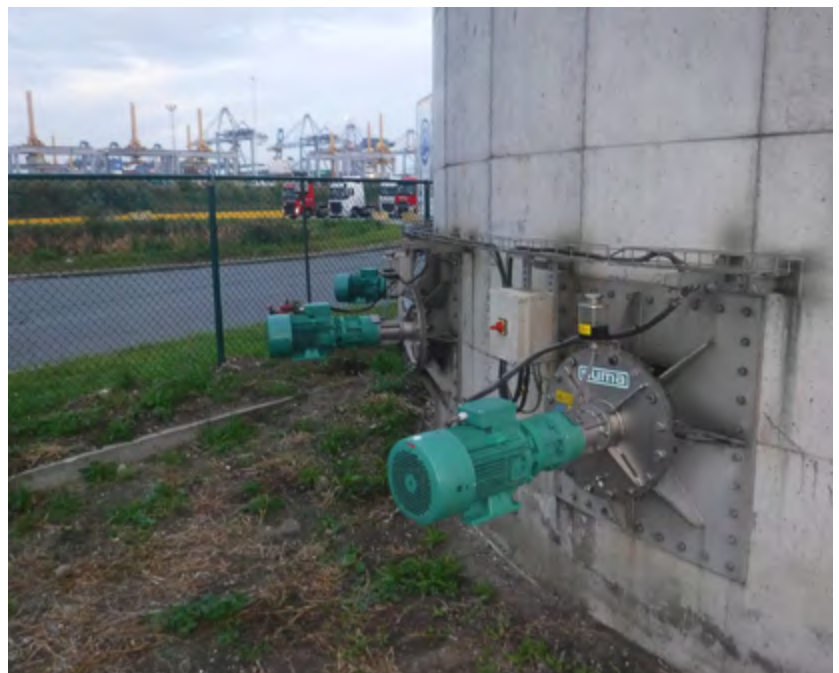
FR light - Concrete tank
