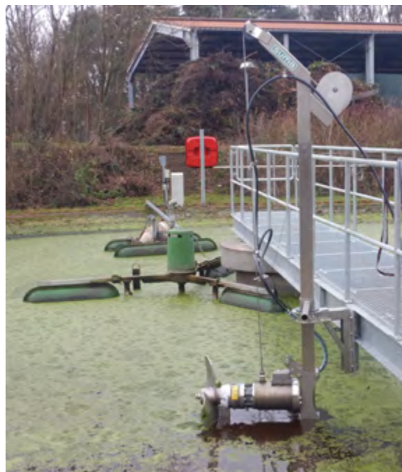
2A with EV - Open tank
