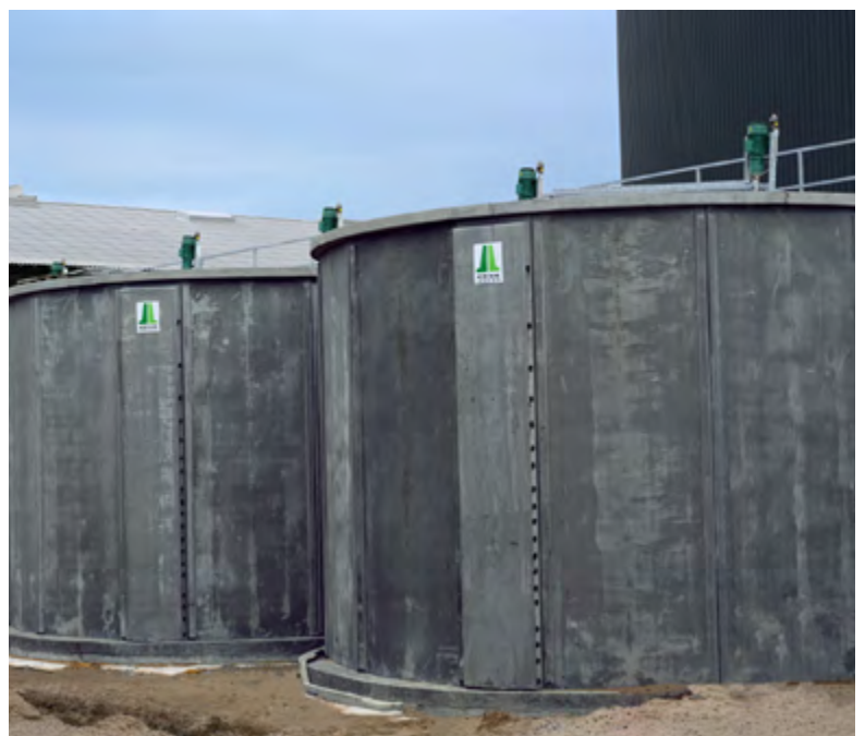
BG2 top mount - Concrete tank
