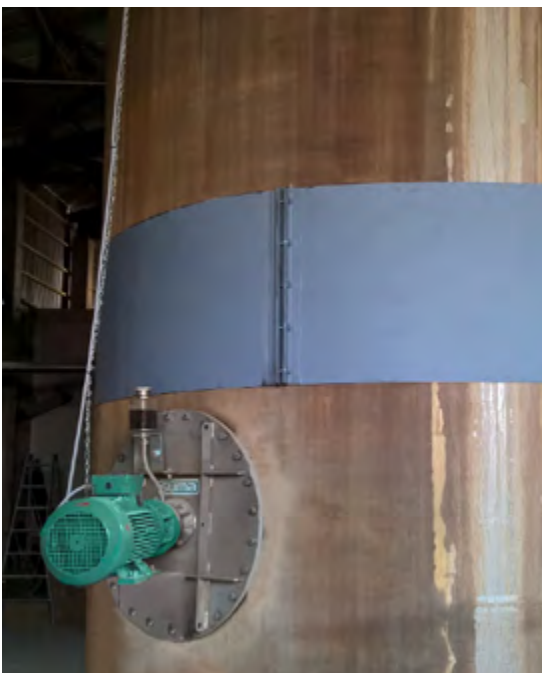
FR light - Steel tank
