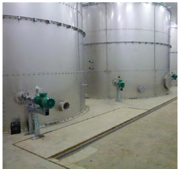
FR stationary - Steel tank
