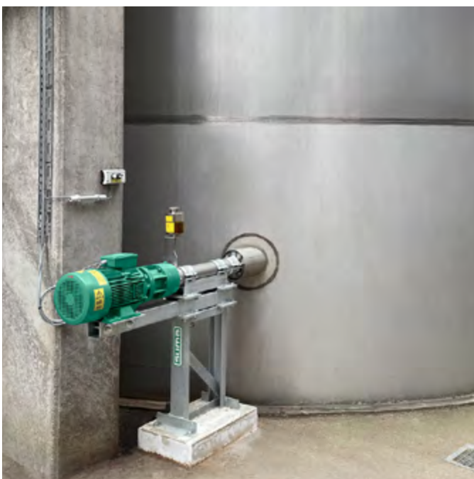
FR stationary - Steel tank
