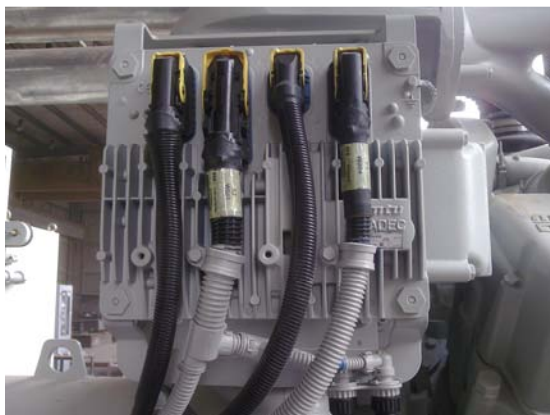
ADEC ECU Mounted on the engine
